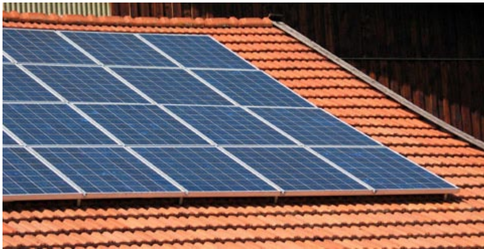
Figure 2 - Example of a roof mounted solar energy system
