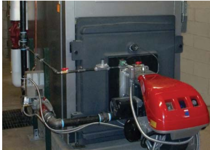
The Vitorond 200 supplements the system with higher temperature water in the winter
