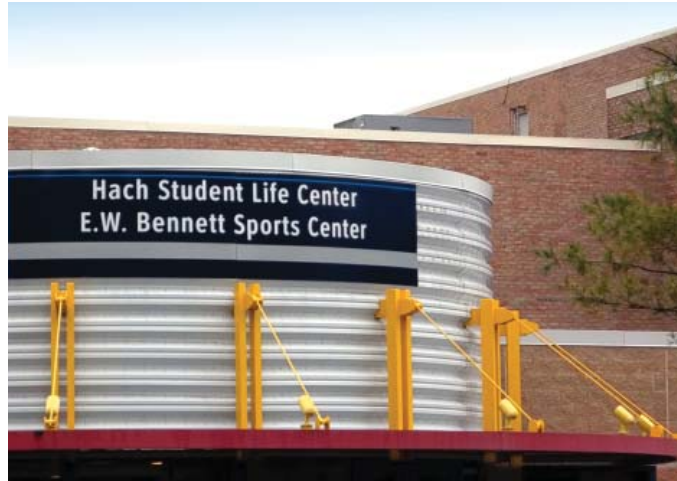
The original boiler was replaced with a more efficient gas-fired hybrid heating system
