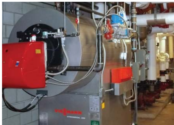
The Vitocrossal 300 serves as lead boiler during the spring and fall to maximize energy savings
